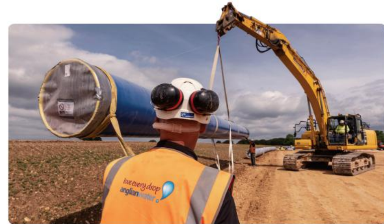
Figure 30 Moving water to supply our customers
