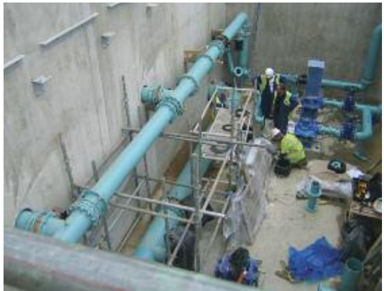
Construction of a new blending tank at our East Dereham Water Treatment Works in Norfolk.
