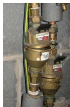
Figure 4: Lack of insulation will allow internal water meters to freeze and split causing a loss of water supply
